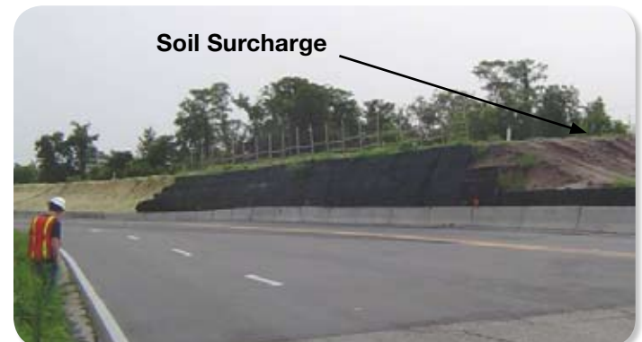
A 28-foot high soil surcharge, similar to this one from a project on another highway will compact the soil within the stabilized depression for several years.
